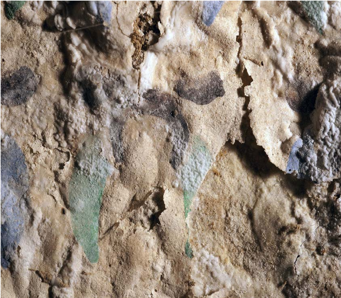
Figure 8: Harm caused by salt in Mogao Cave no. 80.
